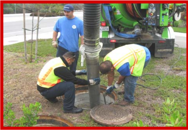
Remove Access Hatches Set Up Vacuum Truck to Clean The Pretreatment Chamber.
