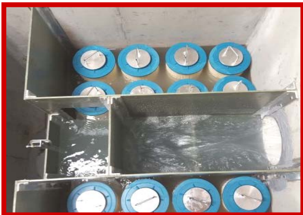
Assess the Condition of the Filter Cartridges and Determine If Cleaning is Required.
