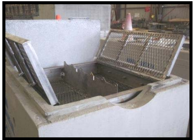
To Replace Media Top of Cage Hinges Open for Unimpeded Access. Vac Truck Can Be Used.
