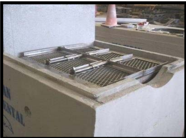
Close Lids of Media Cage. Maintenance of the System is Now Complete.
