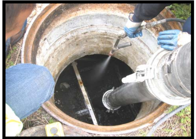
Insert Vacuum Hose in the Sediment Chamber on the Influent End of the System and Vacuum at all Sediment and Standing Water.
