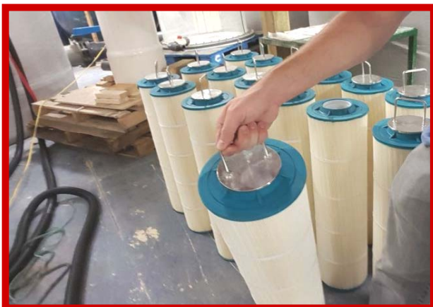
Once Cleaned Install Back Into the Vault. This Completes Maintenance. Ensure Access Lids are Properly Replaced.
